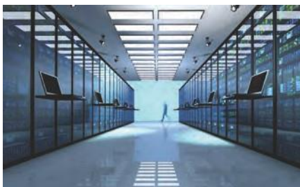
CENTRE DE DATE, CAMERE SERVER
